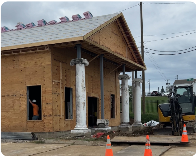
Fire Station No. 1 renovations began in 2024, the 1978 structure remodeled and adding space for administrative offices and women's domicile.
